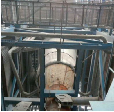
Fig. 1. Site photos of the cyclone separator used in CFBC plant
